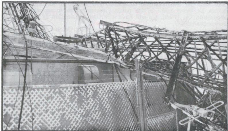
WCEC downed tower laying on equipment building, used for communications between crews and for scada switching.
