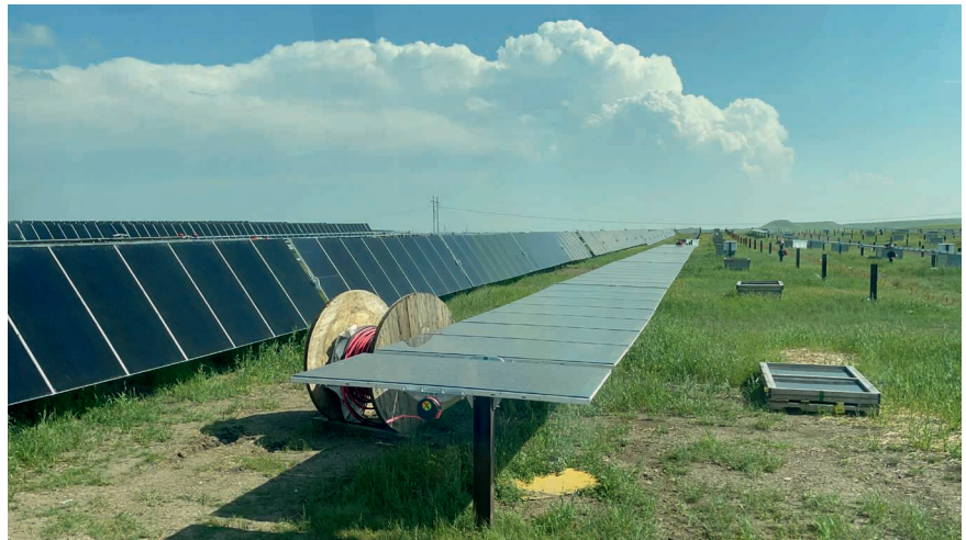
A look on the ground as crews prepare the Wild Springs Solar Project for power generation. Photo submitted by East River Electric
